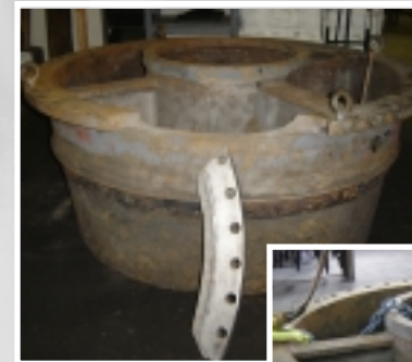
Broken flange on a large cast iron hub
