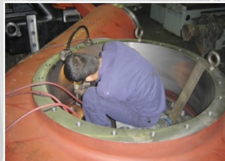
Large turbine scroll with porosity in the machined surface, being repaired by our metal locking process and hand finished back to machined dimensions
