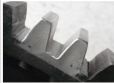
Typical gear tooth repair. Replacement teeth are fabricated, fit and aligned to ensure smooth, tight fit with proper lash
