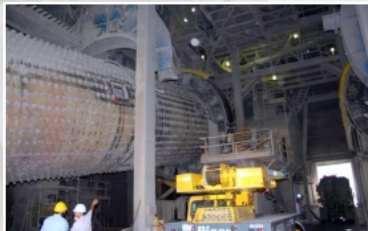
On-site inspection in San Jose, CA of large ball mill that had separated from the drive end trunnion
