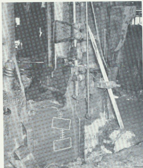
The completed repair showing the inlays installed flush with parent metal, in combination with metal locks. Base is now ready to operate efficiently for many more years.
